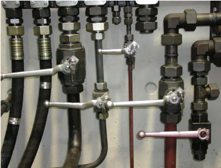
Fig. 3 Securing against unintentional re-closing by lockable ball valves.
