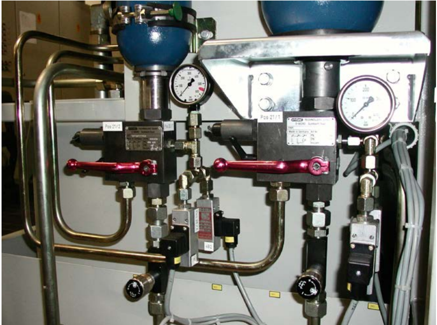
Fig. 25 Depressurized hydraulic accumulators with closed pressure lines
