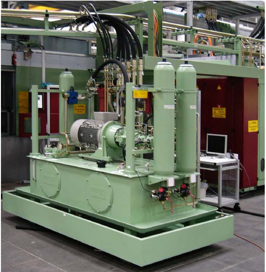
Fig. 24 Hydraulic power unit on stationary production facility
