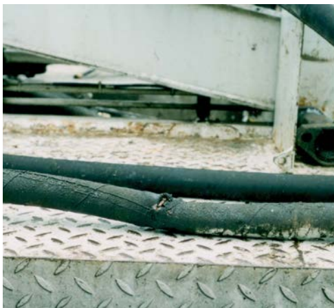
Fig. 2 Bursted hydraulic hose assembly
