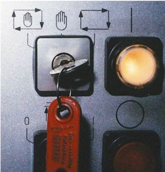
Fig. 26 Mode selection switch at machine control desk [H]
