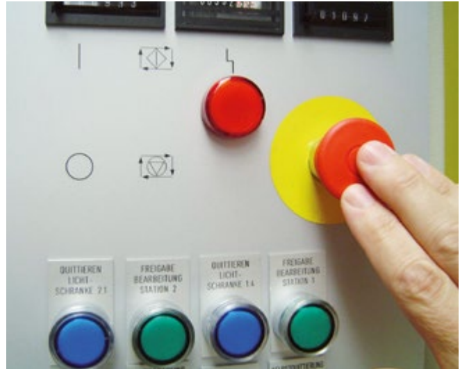
Fig. 32 Emergency-stop control device at a robot system [H]
