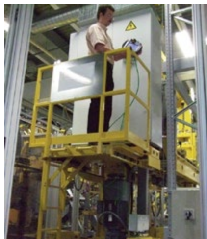
Fig. 59 Fixed access to the control cabinet with ladder and platform [H]
