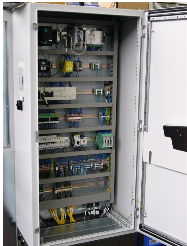
Figure 11: Open control cabinet of a test bench
