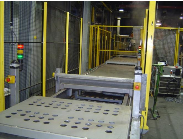
Figure 3: Assembly of machinery in trial operation with partly erected protective fence; emergency switch off circuits and visual warning devices are already operational
