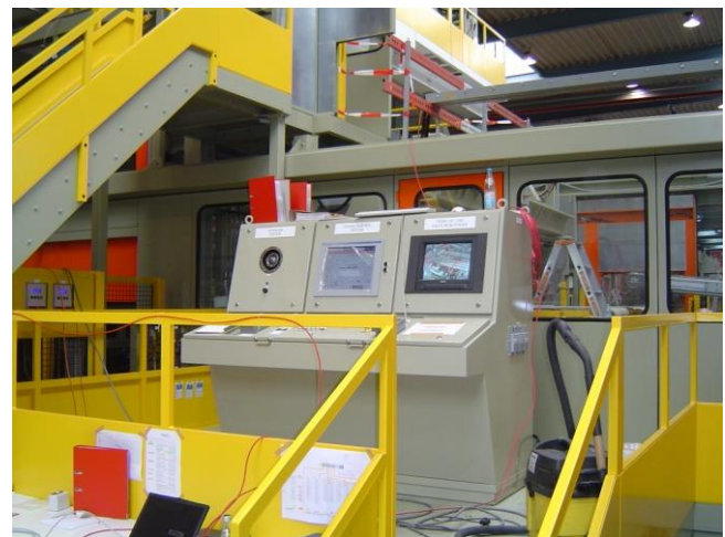
Figure 4: Control station with video surveillance
