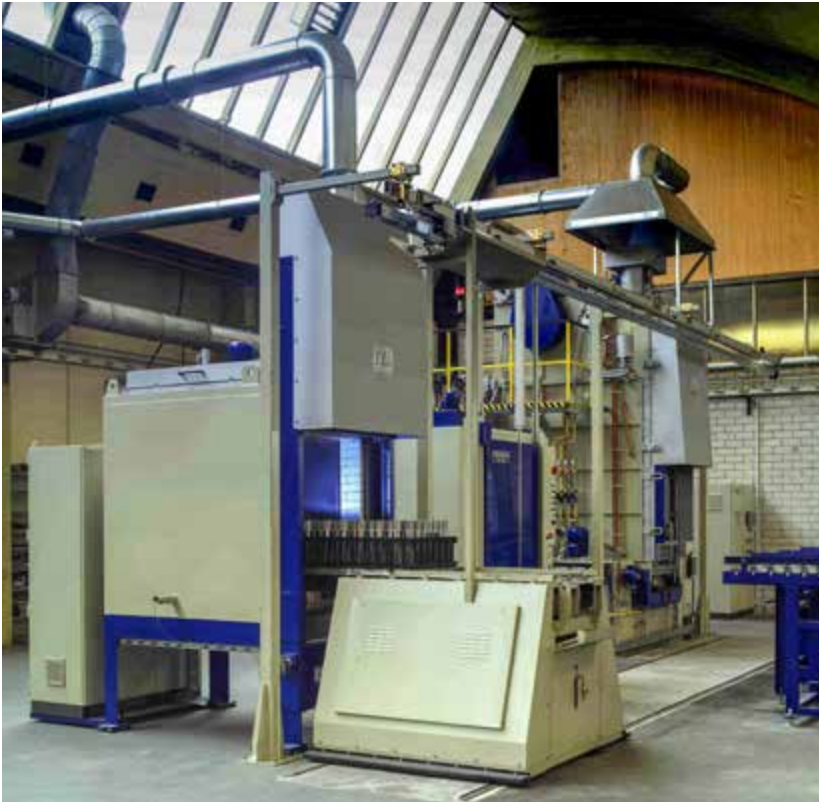
Figure 36 Multi-purpose chamber furnace line comprising tempering furnace, cleaning plant and multi-purpose chamber furnace
