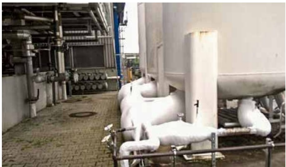
Figure 31 Formation of ice on nitrogen tank pipelines
