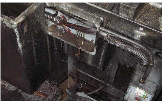
Figure 4: Scorched exposed cables
