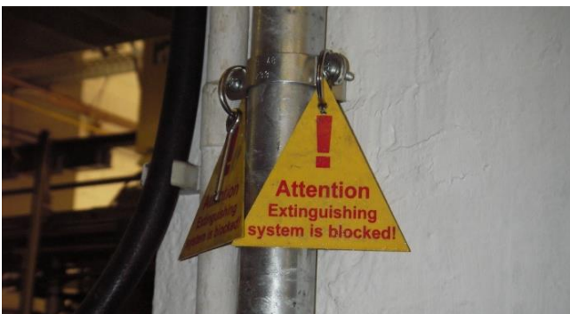
Figure 3: Blocking of the fire suppression system
