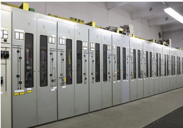
Fig. A 5-17 High-performance switchgear of older design; intended for industrial use
