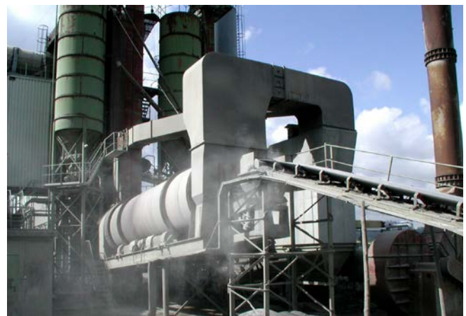
Figure 10: Dry drum of an asphalt mixing plant
