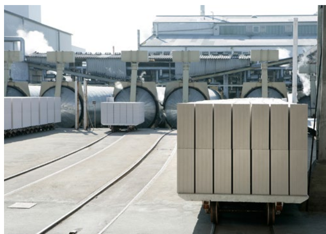
Figure 17: Exit area of hardening boilers for sand-lime bricks. Source: VBG
