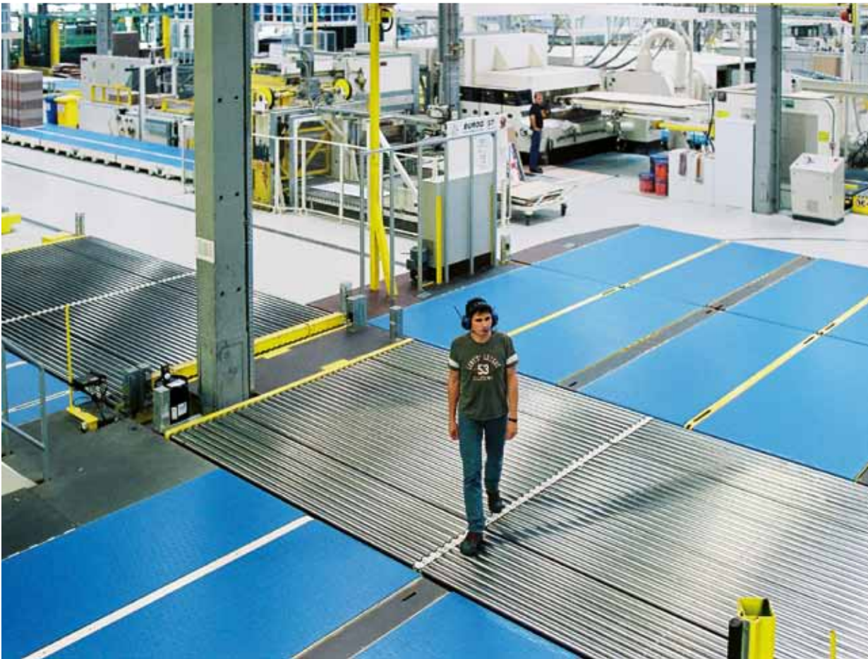
Ideally all spaces between the conveyors are lined with filling plates. Thus, tripping areas can be defused.
