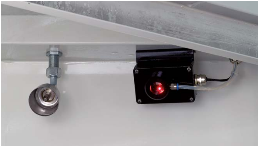
Figure 53 Fire detection elements (optical sensor) with purging air
