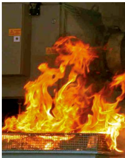
Figure 44 After-Fire subsequent to extinguishing
