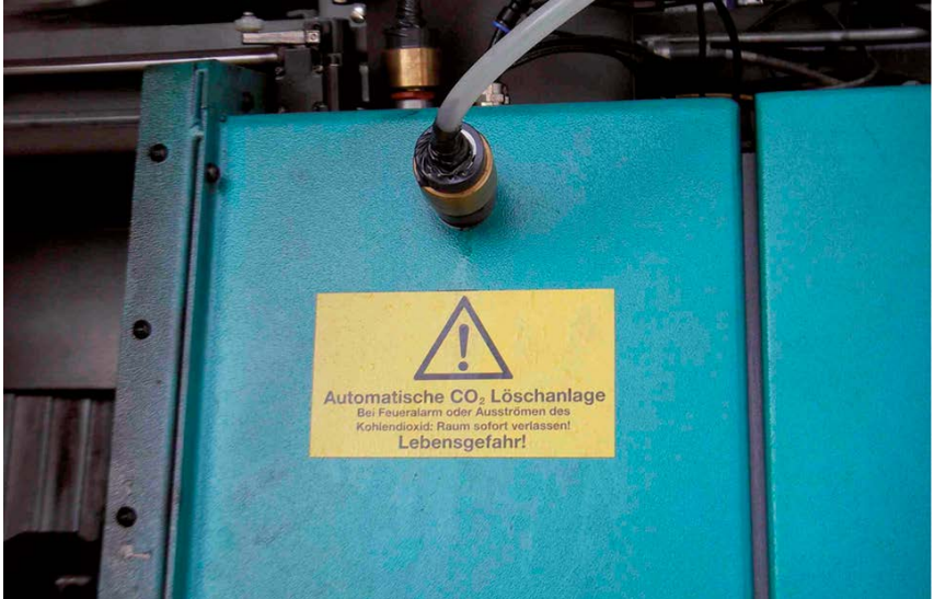
Figure 58 Warning sign for CO 2 extinguishing gas hazards
