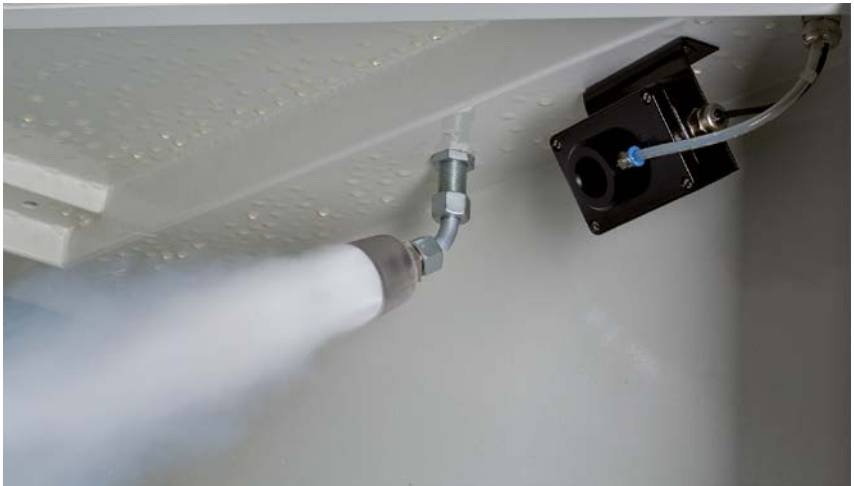
Figure 54 Extinguishing nozzle in operation
