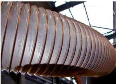
Figure 36 Accumulation of oil in the extraction ducting
