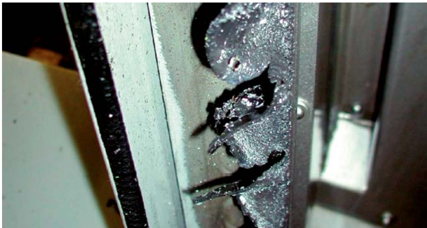
Figure 28 Door sealing not suitable for technical fire prevention and protection
