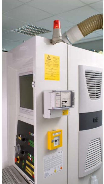
Figure 52 Fire alarm centre with manual activation
