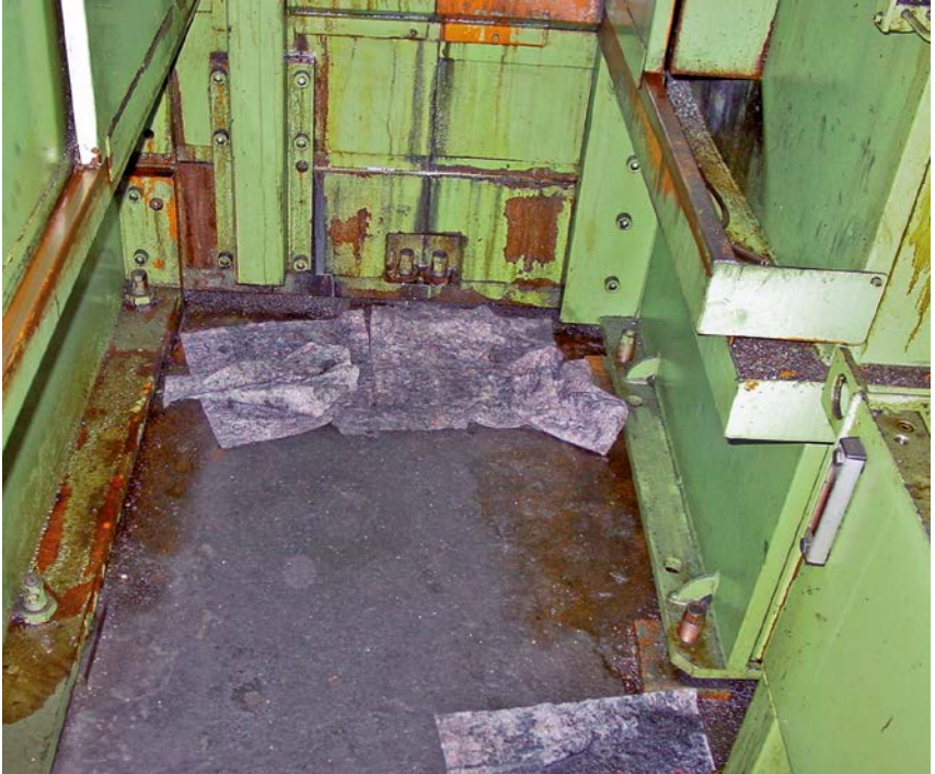
Figure 57 Fire hazard near to a machine
