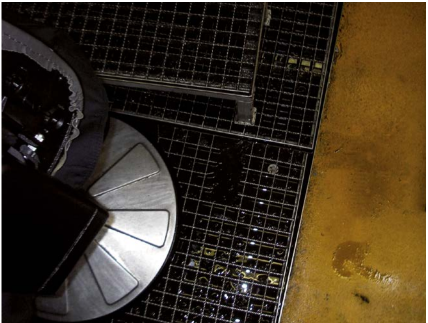
Figure 55 Oil-filled gratings with large surface areas
